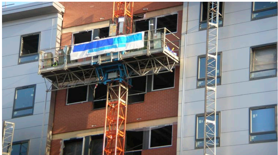
Figure 14 A mast climbing work platform
