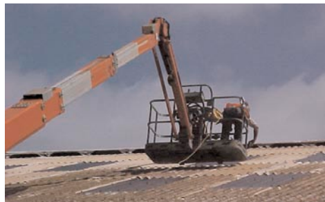
Figure 26 A mobile elevating work platform being used to replace a roof sheet
