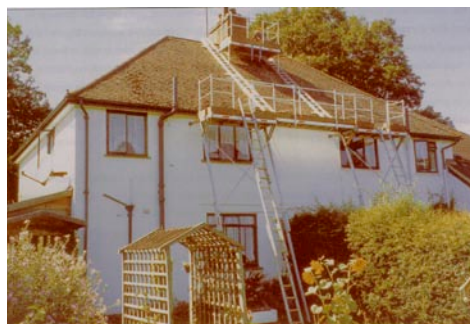
Figure 25 Proprietary access system for roof-work
