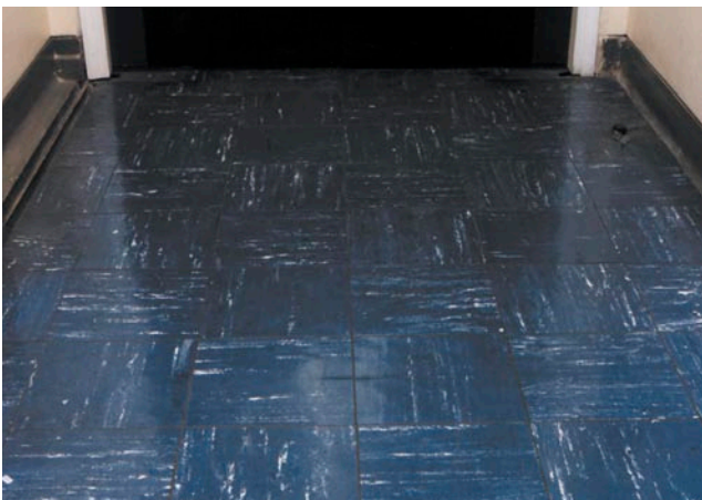
Figure 48e Asbestos-containing vinyl floor tiles
