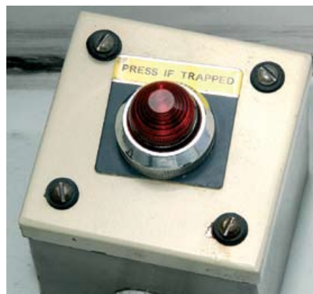
Figure 55 Trapped man alarm
