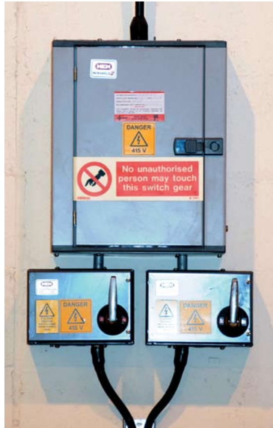
Figure 10 Isolation switch for fixed equipment
