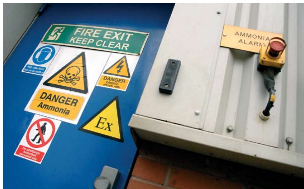
Figure 56 An ammonia plant room emergency exit and alarm
