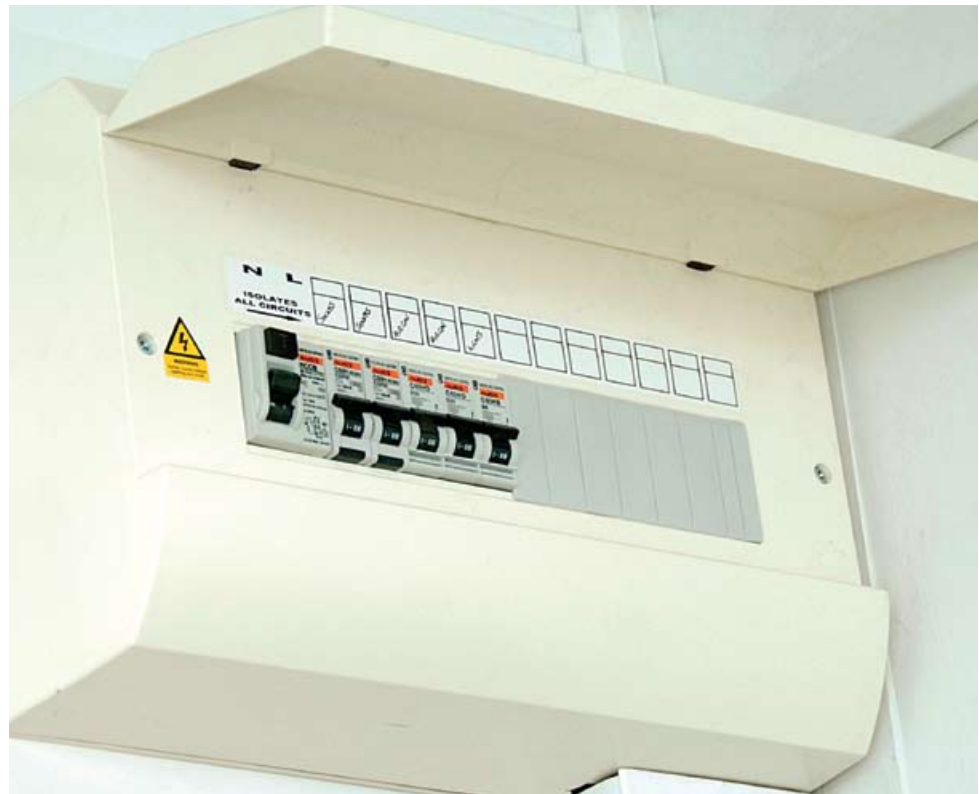
Figure 9 An RCD in a distribution board
