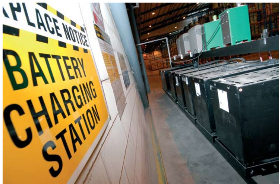
Figure 20 Battery charging station
